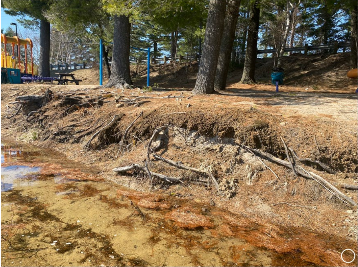
Figure 4. Example of shoreline erosion
