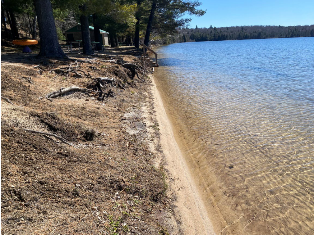
Figure 1: Exposed tree roots within shoreline slope.
