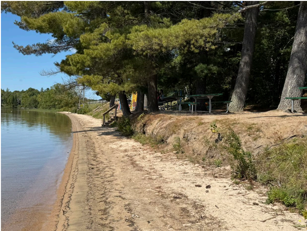
Figure 2: Leaning tree and erosion of toe of shoreline slope.
