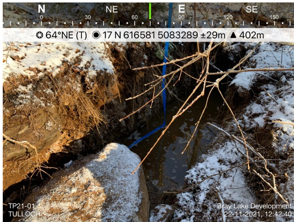
Photo 2: TP21-01 note large boulders in test pit at time of investigation.
